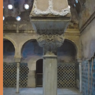
Salt damage affecting the Baños de Comares at the Alhambra, Granada (Spain). PHOTO: E. SEBASTIAN PARDO
